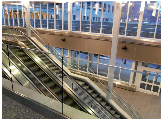
Base shoe glass railing with top cap on stair and balcony.
