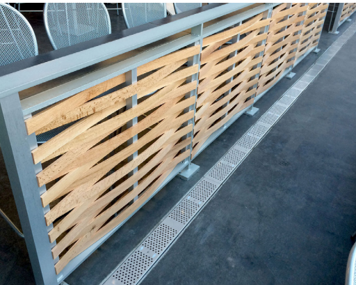
Custom aluminum framed railing with wood infill in the upper level (Minnie and Paul's).
