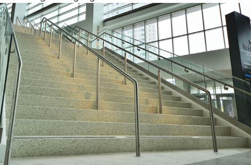
LED lighting incorporated into handrails on stairs and intermediate aisles.
