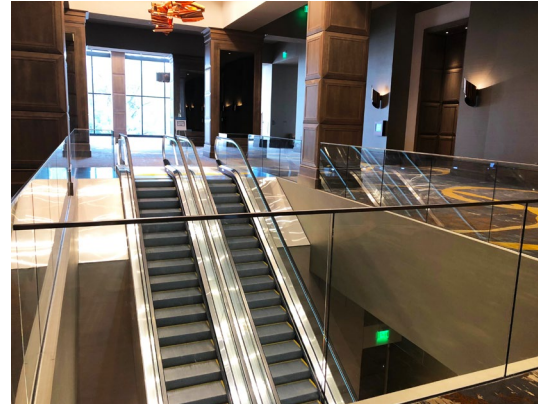
The escalator that guides visitors to the lower level art gallery is lined with custom guardrail featuring SGP laminated glass.
