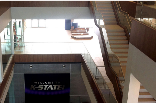
Base Shoe balcony glass railing in 4-story atrium.
