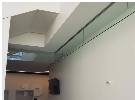
350 LF of glass smoke baffle was installed at the suite and upper club level of the arena.
